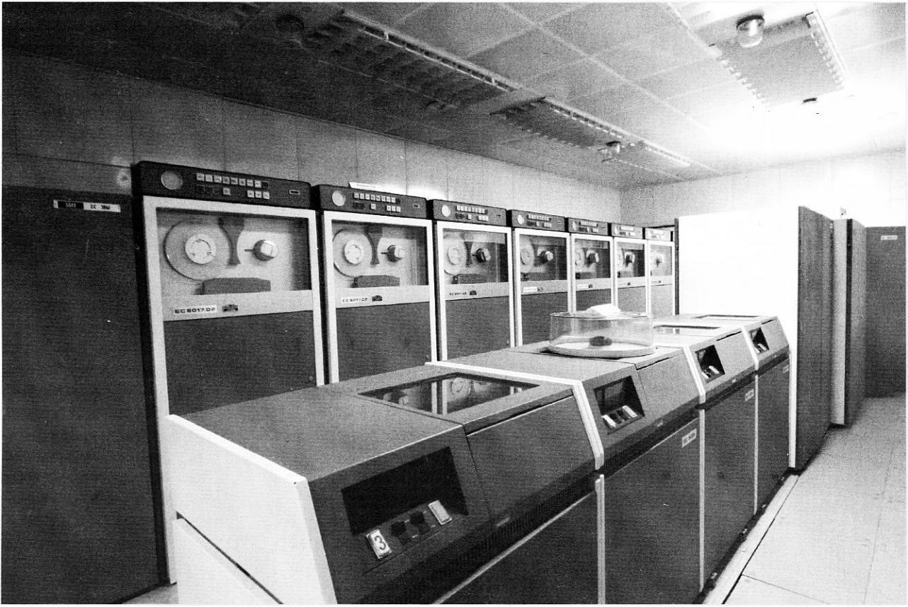
The computer and data centre
